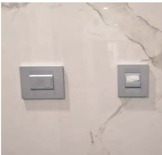
Devices inside the Nobakht building
