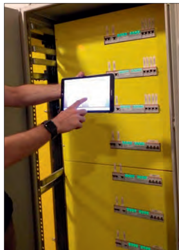
Cabinet operation being controlled by tablet interface.
