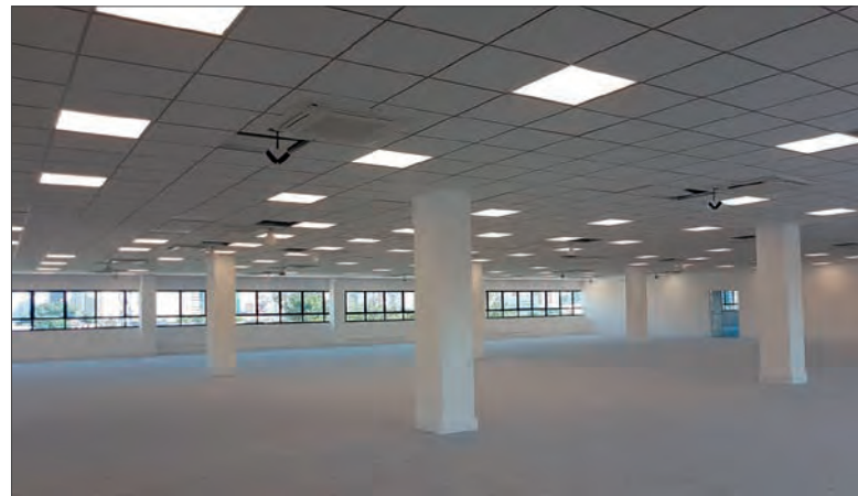
Efficient control of 1600 lighting ballasts is provided.
